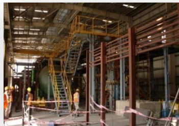
COLOUR COATING LINE FOR TATA BLUESCOPE LTD.
