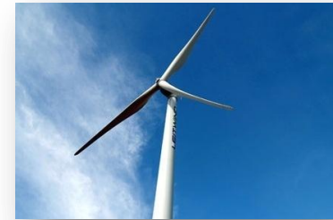
1.5 MW WIND TURBINE AT UTHUMALAI
