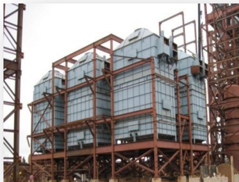
COAL GASIFICATION PLANT FOR JINDAL STEEL
